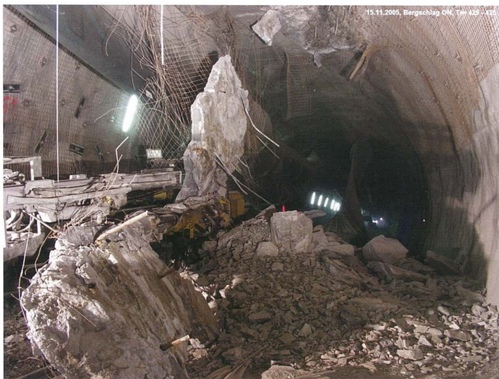
Figure 2. Damage caused by a rock burst event
